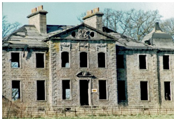
1988: Note the slate-stripped roof and gaping windows
